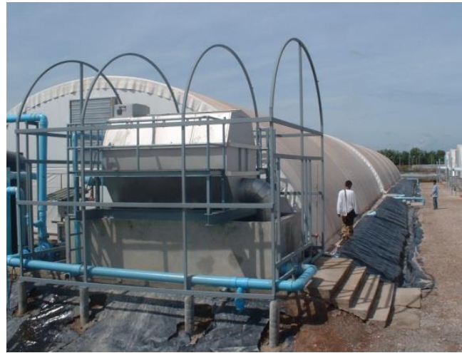
The outlet water is fed to a drum filter, bio-filter
