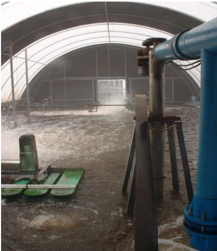
Poly-tunnel shrimp pond with circulation and central outlet pipe
